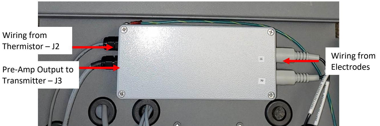
Figure 10. Pre-amplifier located behind the wet panel.
